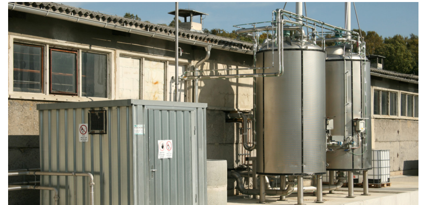
Figure 6.3-3: Pilot biogas plant Fraunhofer IKTS
